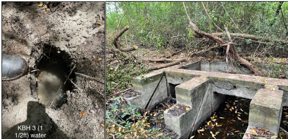
Figure 50 - 5.24: Shallow Water Table (left); Debris Blocked and Structurally Damaged Sluice Canal.
